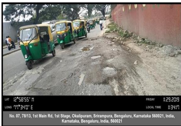
Fig 4: Poor condition road fully deteriorated
